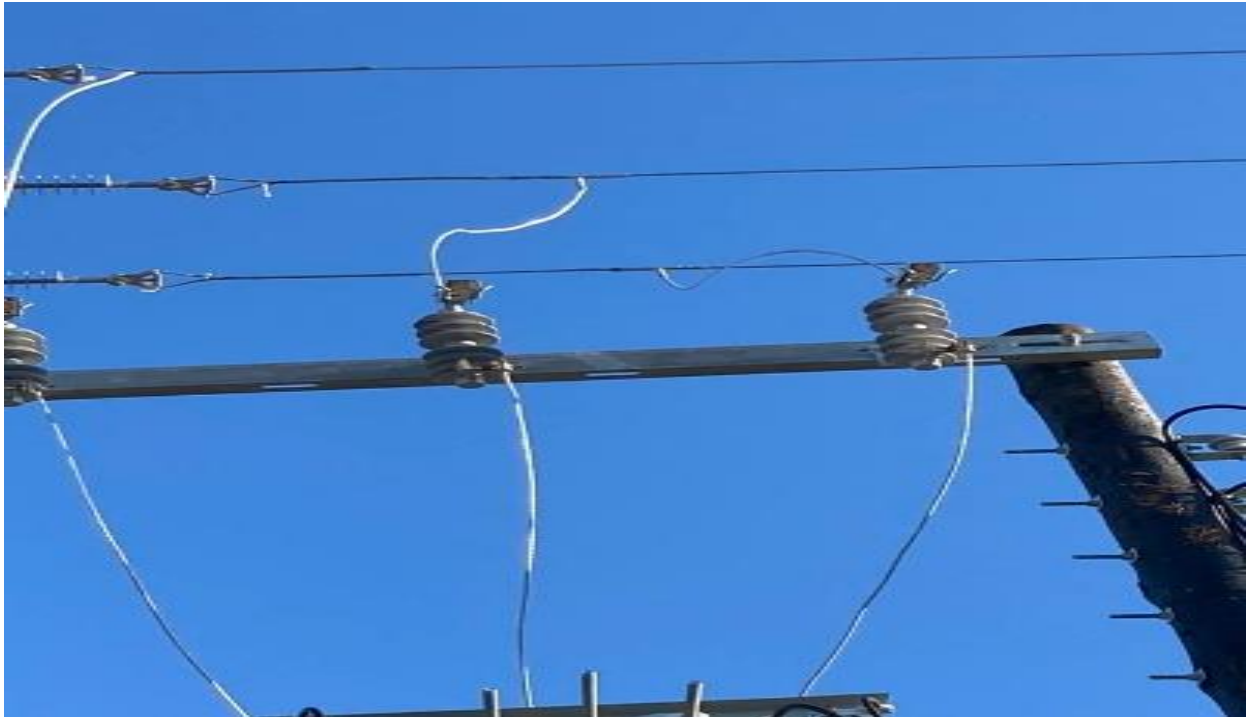
Figure 19: Transformer protection fuses
