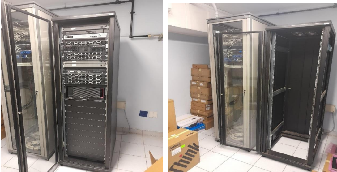
Figure 129: Disaster Management server room
