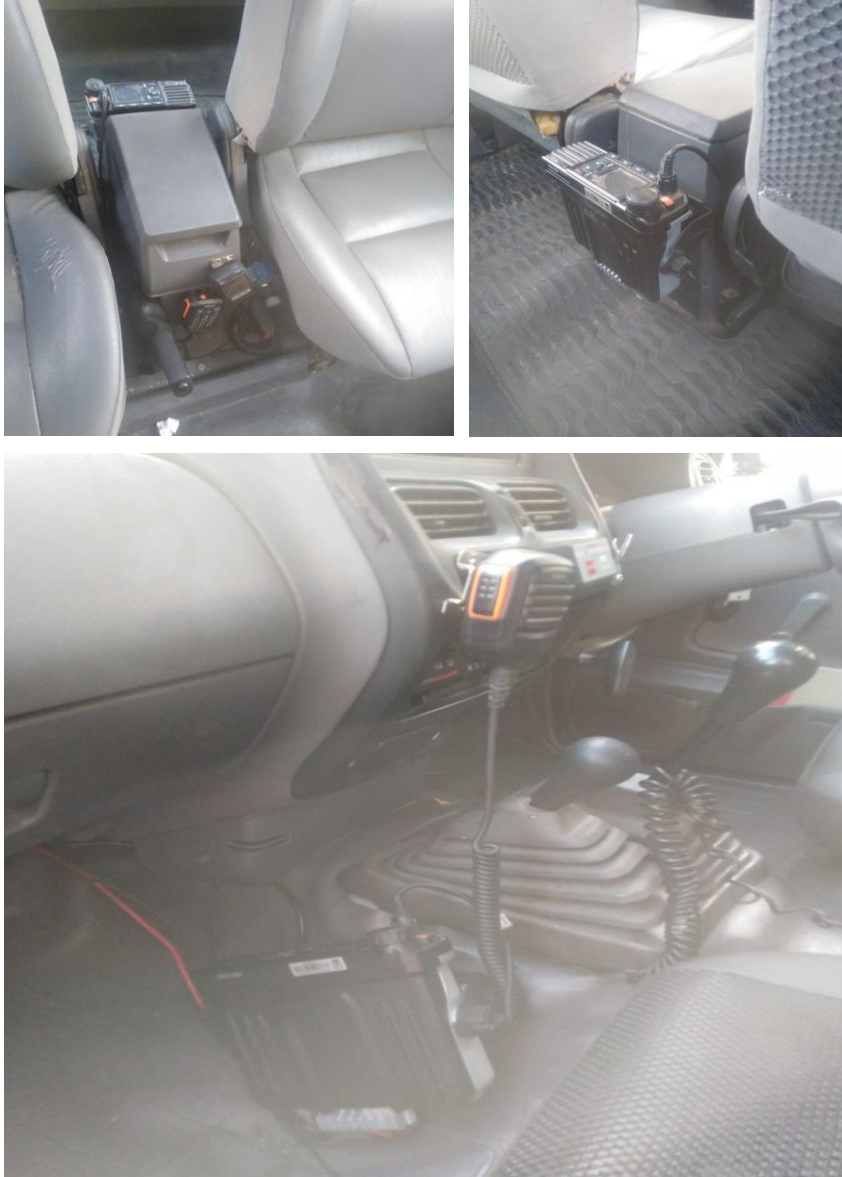
Figure 134: Mobile radios installed in Fire and Disaster Management vehicles
