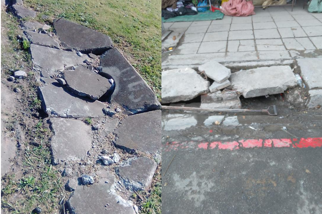
Figure 25: Damaged kerb inlets
