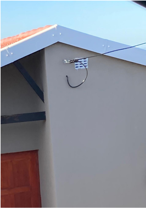
Service Connection entering dwelling
