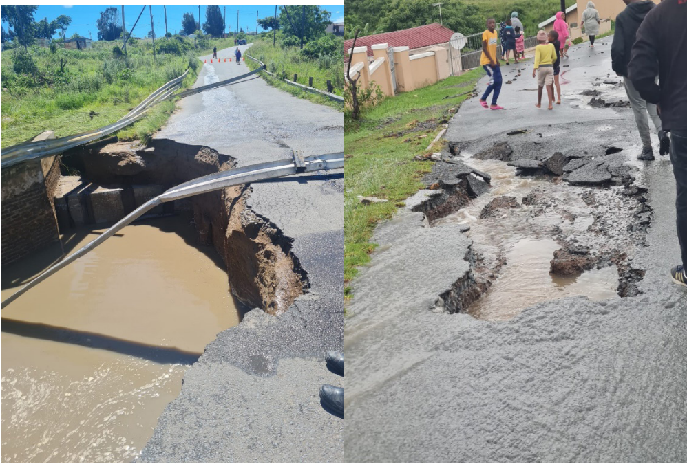
Above: January 8 Flooding
