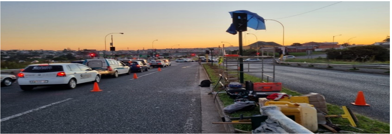
Figure 11 New Red Traffic Light camera installation
