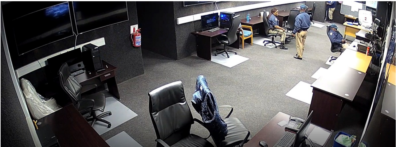
CCTV Monitoring Hall T3.20.7
