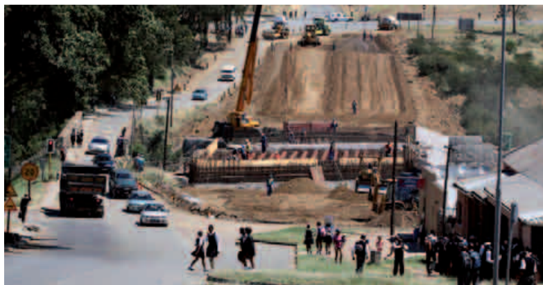
Construction work is underway to build a R26 million bridge and a second lane for traffic into Breidbach.
