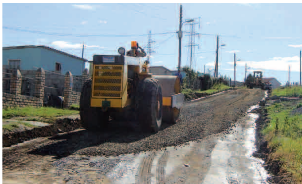
Road construction and maintenance will be one of the key service delivery projects in the metro.
